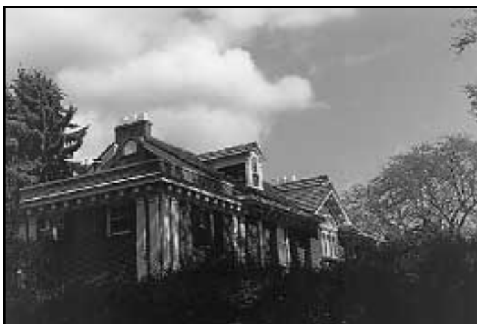
Highly textured roof materials are a character defining feature of the district.
